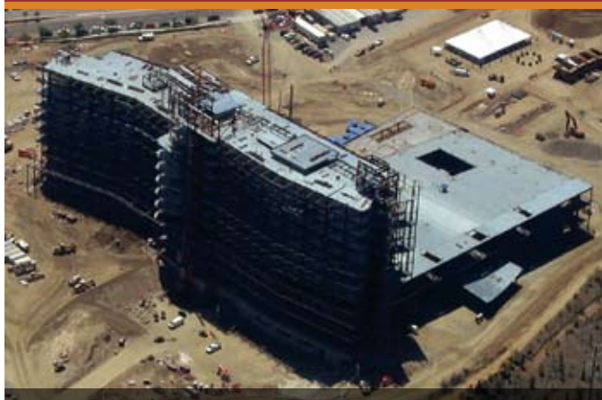
Aerial view of the new Palomar Medical Center West construction site – July 2009.
